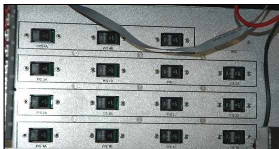
Circuit Breaker Panel
