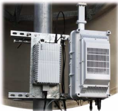
C-Band High power Block Up Converter system
